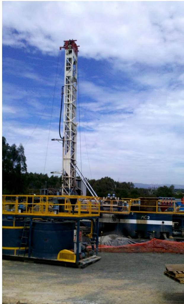
Close up view of Yallourn Power 1 top hole rig (Drilltec Bournedrill TD 2500)
