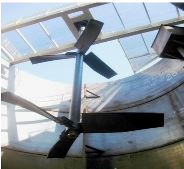
Figure 1: Examples of Agitators for CIL Tanks
