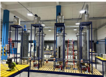
Figure 5 – CCD circuit all plumbed up
