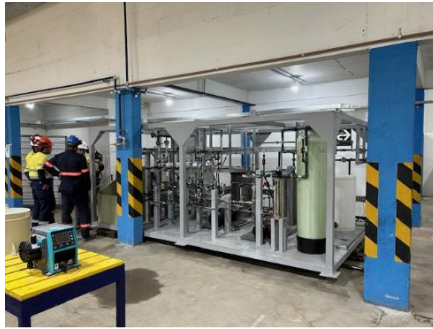
Figure 8 – Water Treatment skid installed
