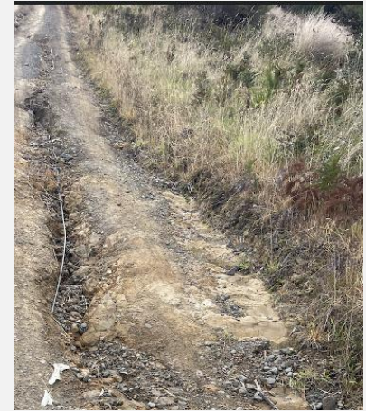
Exposed cable detection
