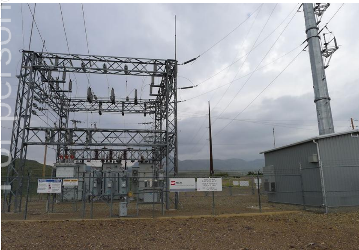
Figure 5: Shafter Mine and Processing Substation.
