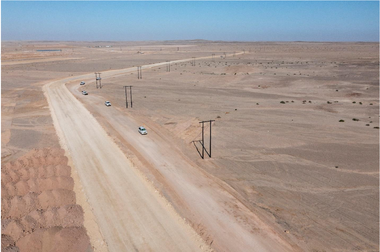
Figure 3: The electrical infrastructure currently under development will support both construction and operational activities on-site. The Etango Project will benefit from a highly reliable power supply sourced from the local grid.
