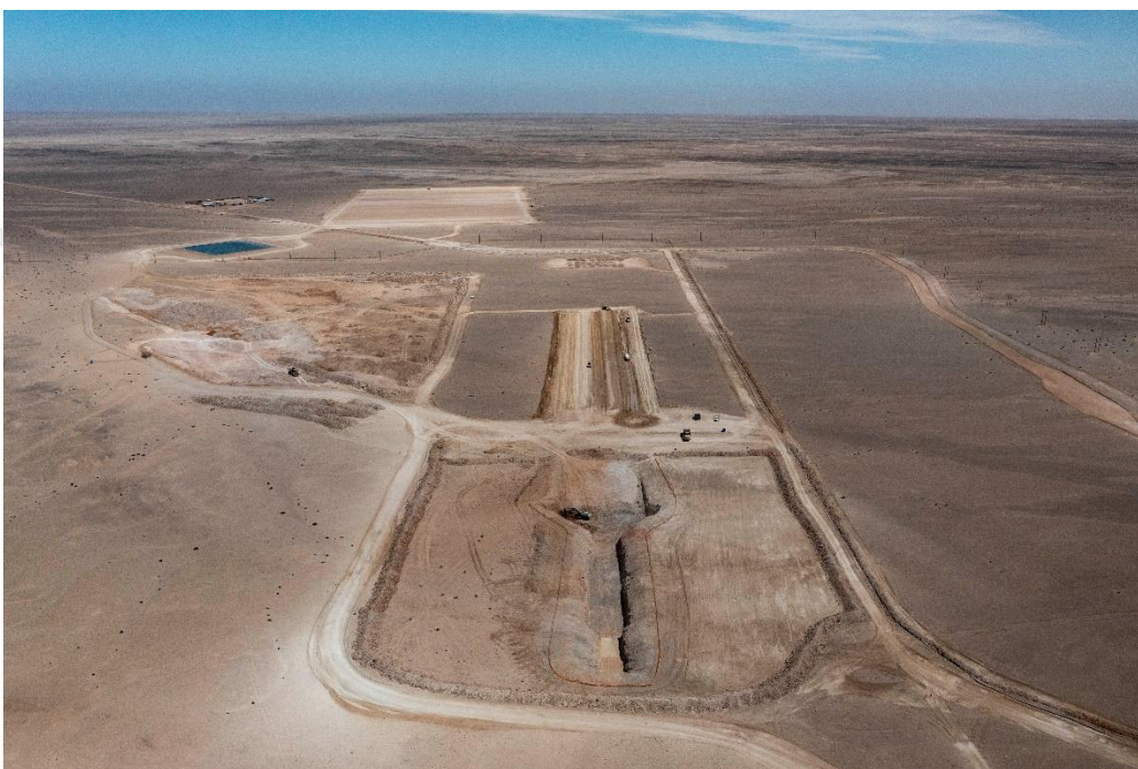
Figure 1: Significant progress continues on bulk earthworks at Etango, a key enabler of future construction and development activities. The primary crusher has been fully excavated and its dimensions confirmed, while work advances on the permanent road and conveyor belt line to the secondary and tertiary crushing areas.
