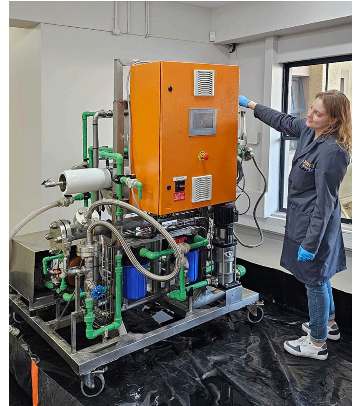
Waste-Water equipment trials, PSG Demonstration Facility
