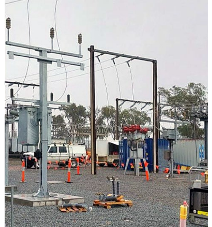
Upgraded Cleve Substation
