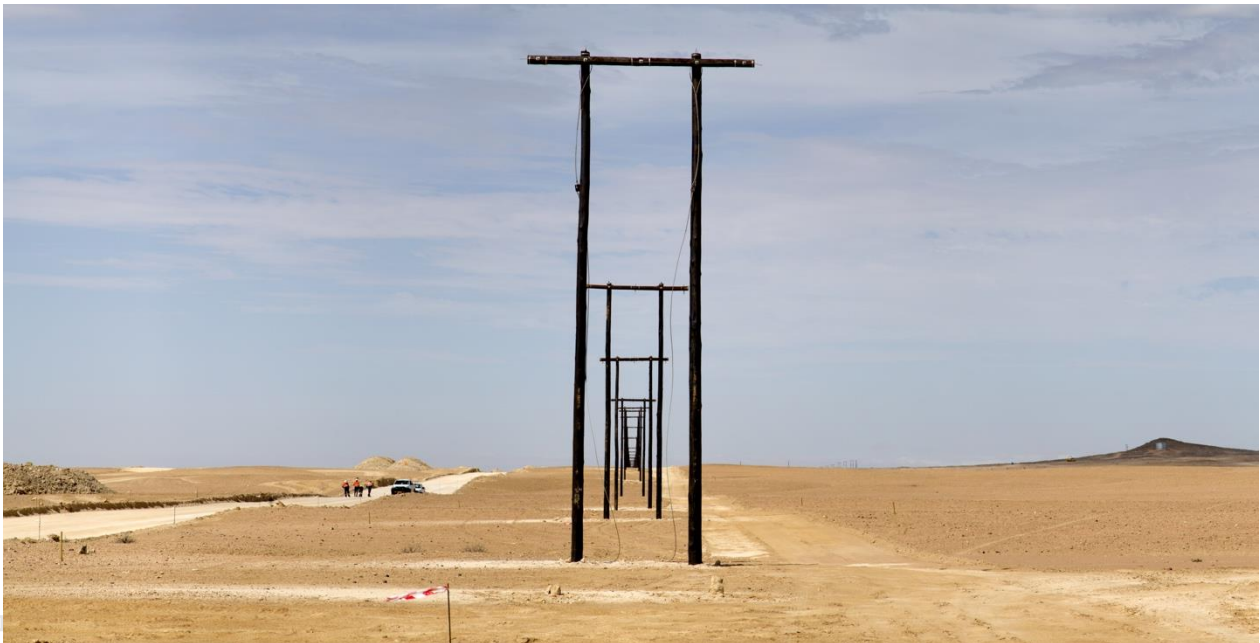
Figure 2: The electrical infrastructure currently under development will support both construction and operational activities on-site. The Etango Project will benefit from a highly reliable power supply sourced from the local grid.
