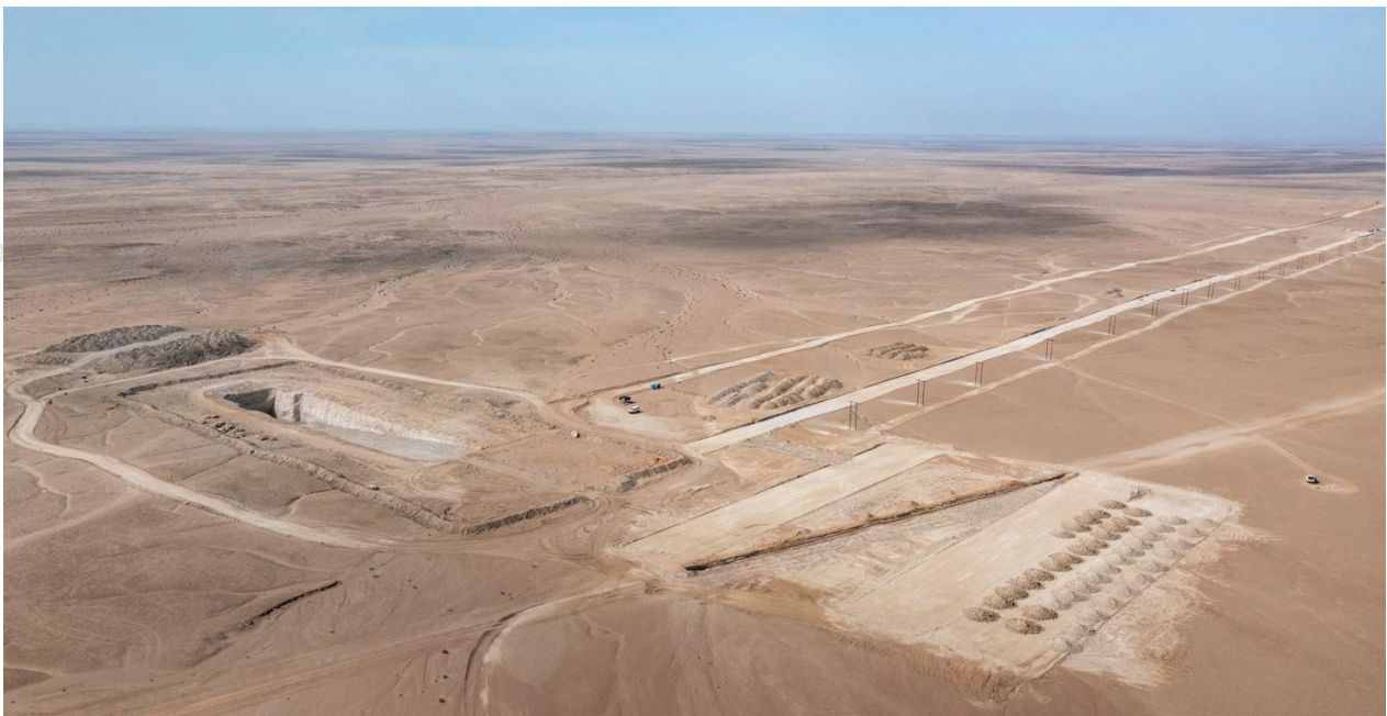
Figure 1: Significant progress continues on bulk earthworks at Etango, a key enabler of future construction and development activities. The primary crusher has been fully excavated and its dimensions confirmed, while work advances on the permanent road and conveyor belt line to the secondary and tertiary crushing areas.
