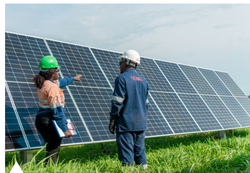
Balama solar and photovoltaic array
