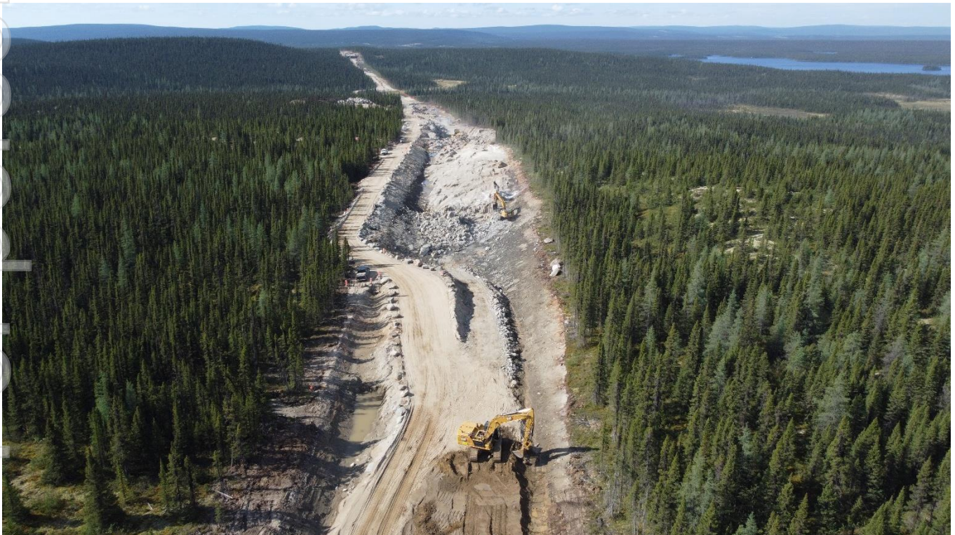
Image 1 – Quebec Department of transport photograph 6 - Highway 389 New route to Fermont that will link with the Lac Carheil Graphite project claims area (Figure 3).
