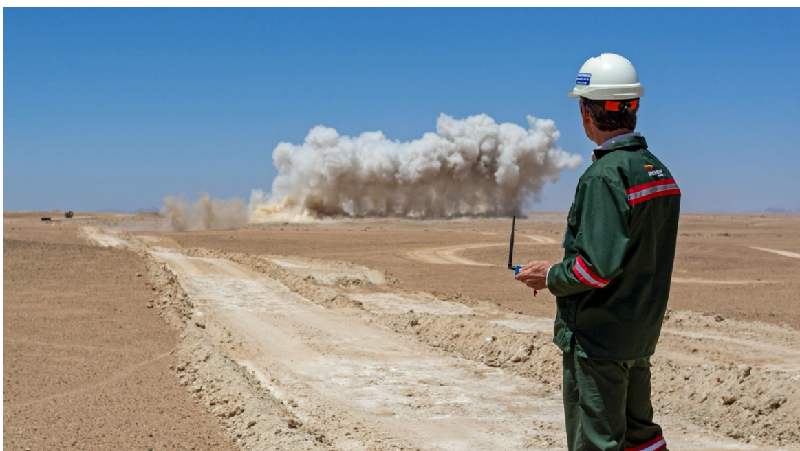
Figure 3: First blast being set off by Bannerman Mining Resources (Namibia) Managing Director, Mr Werner Ewald
