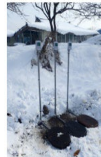
Water meters in underground pits with added communication capability
