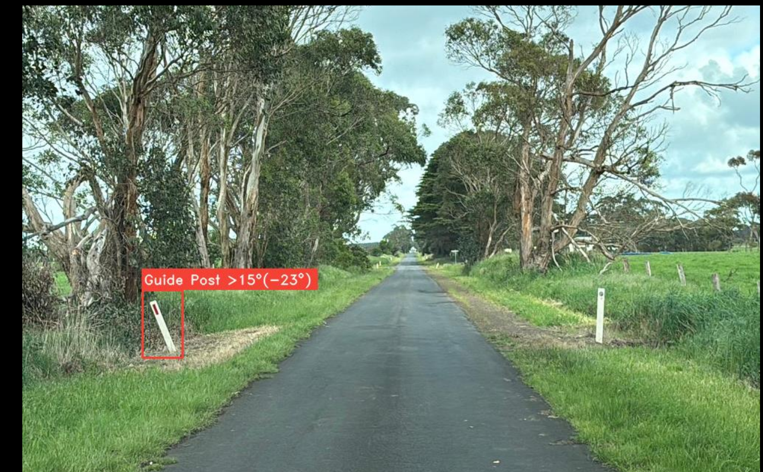
Detection for leaning guide post defects
