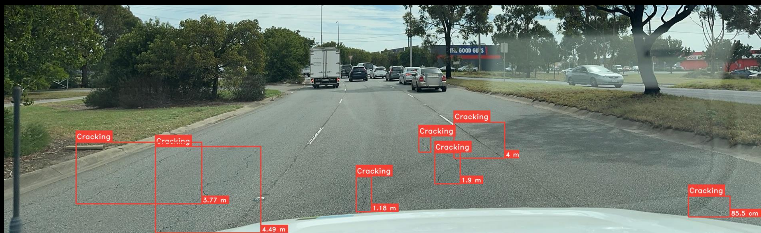
AutoPilot+AI now uses LiDAR to provide approximate measurements of detected defects
