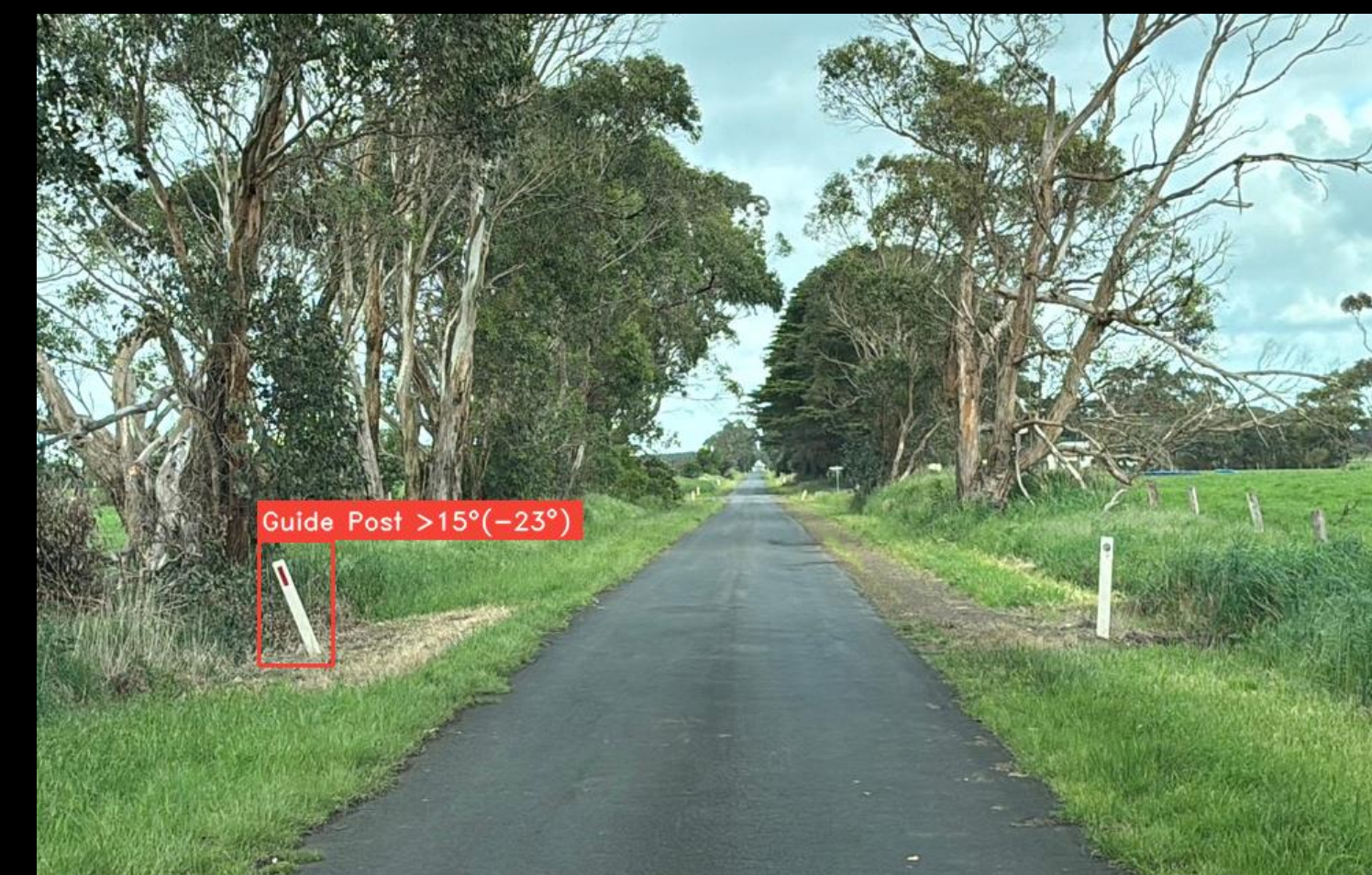
Detection for leaning guide post defects
