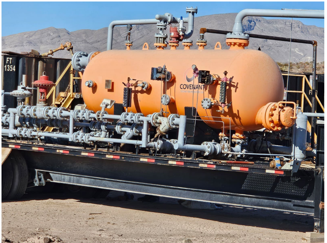
Hydrocarbon Separator at 5201
