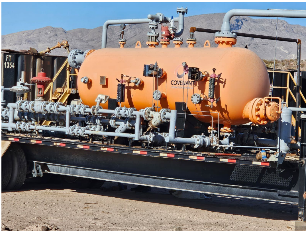
Hydrocarbon Separator at 5201
