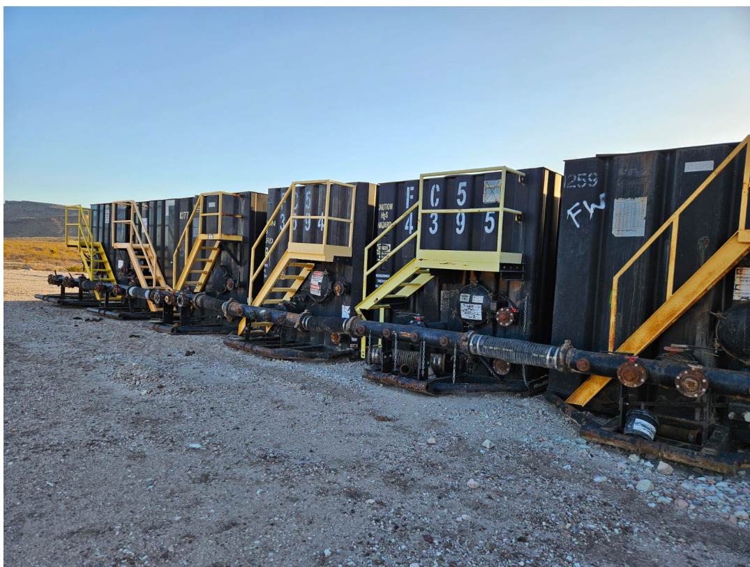
Temporary Water Storage Tanks at 141-2
