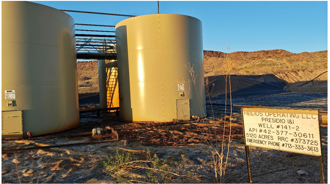
Presidio Well 141 Lease Water and Oil Storage Tanks
