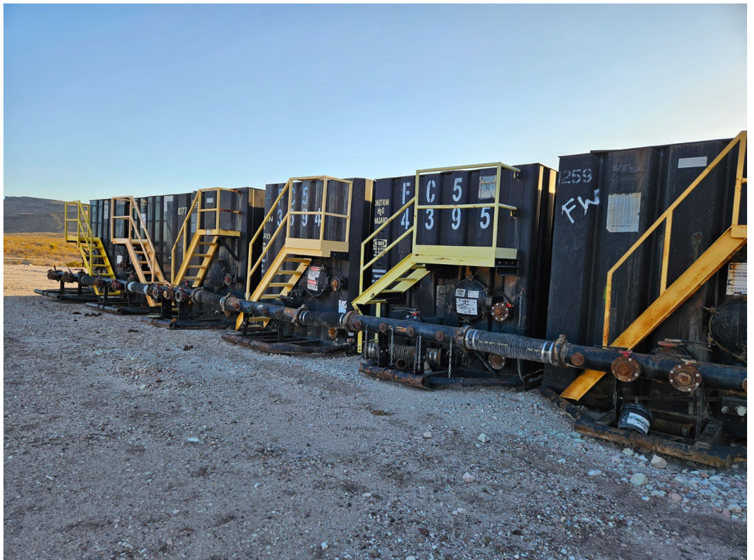
Temporary Water Storage Tanks at 141-2
