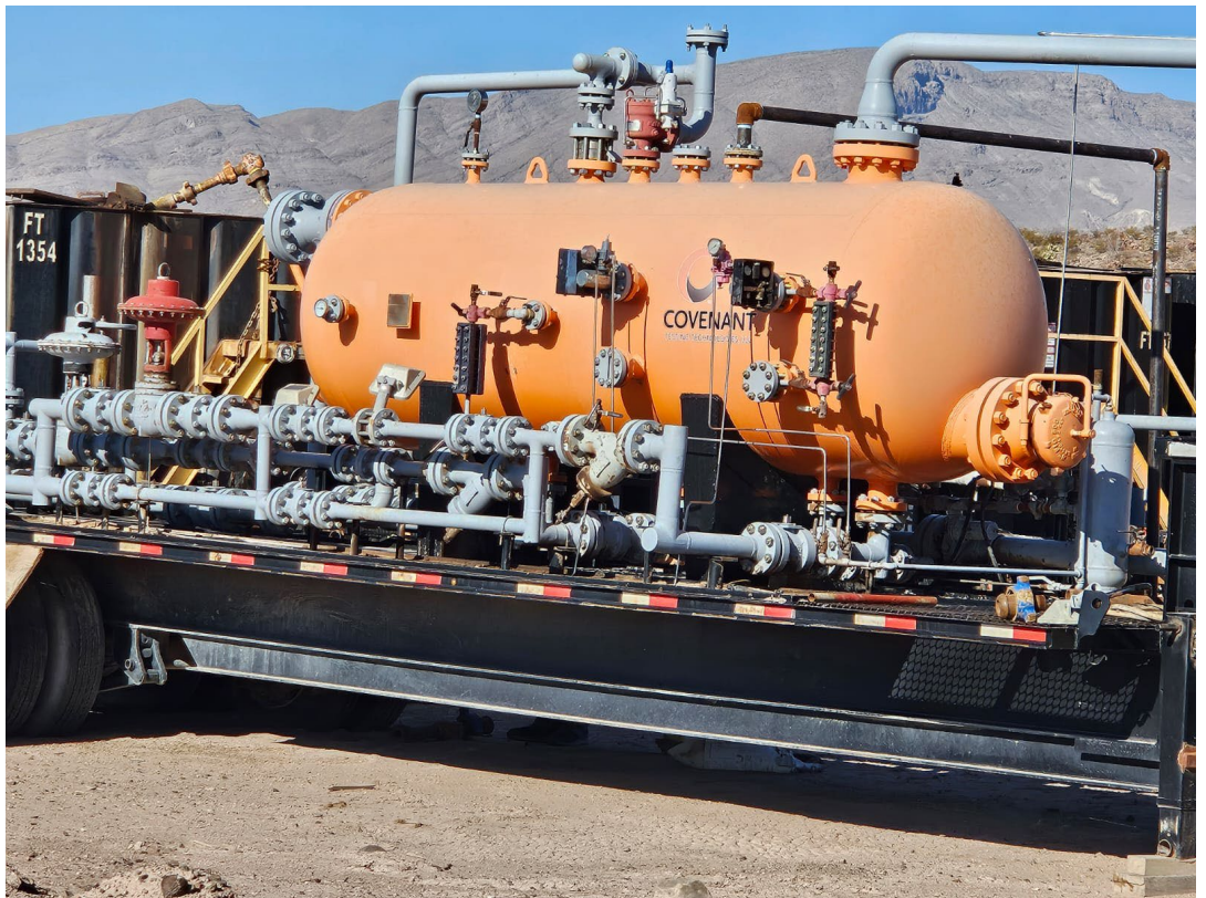
Hydrocarbon Separator at 5201
