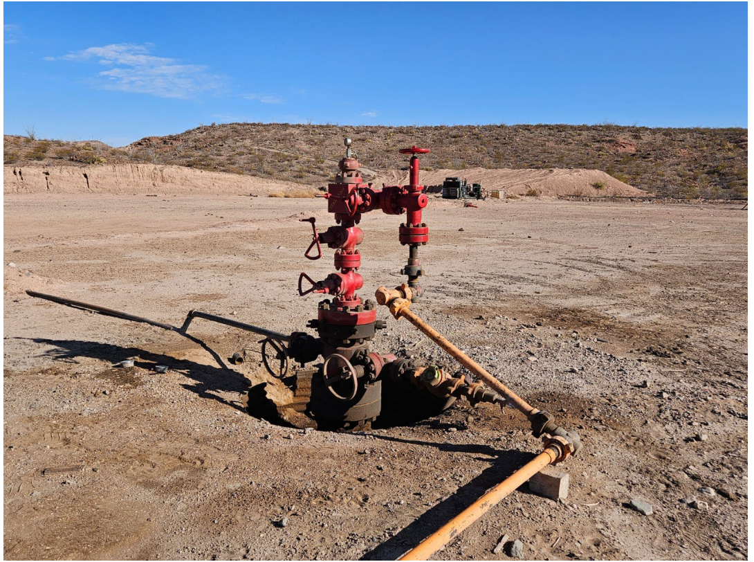
Well Head, Production Tree and Rental Flowline at 5201
