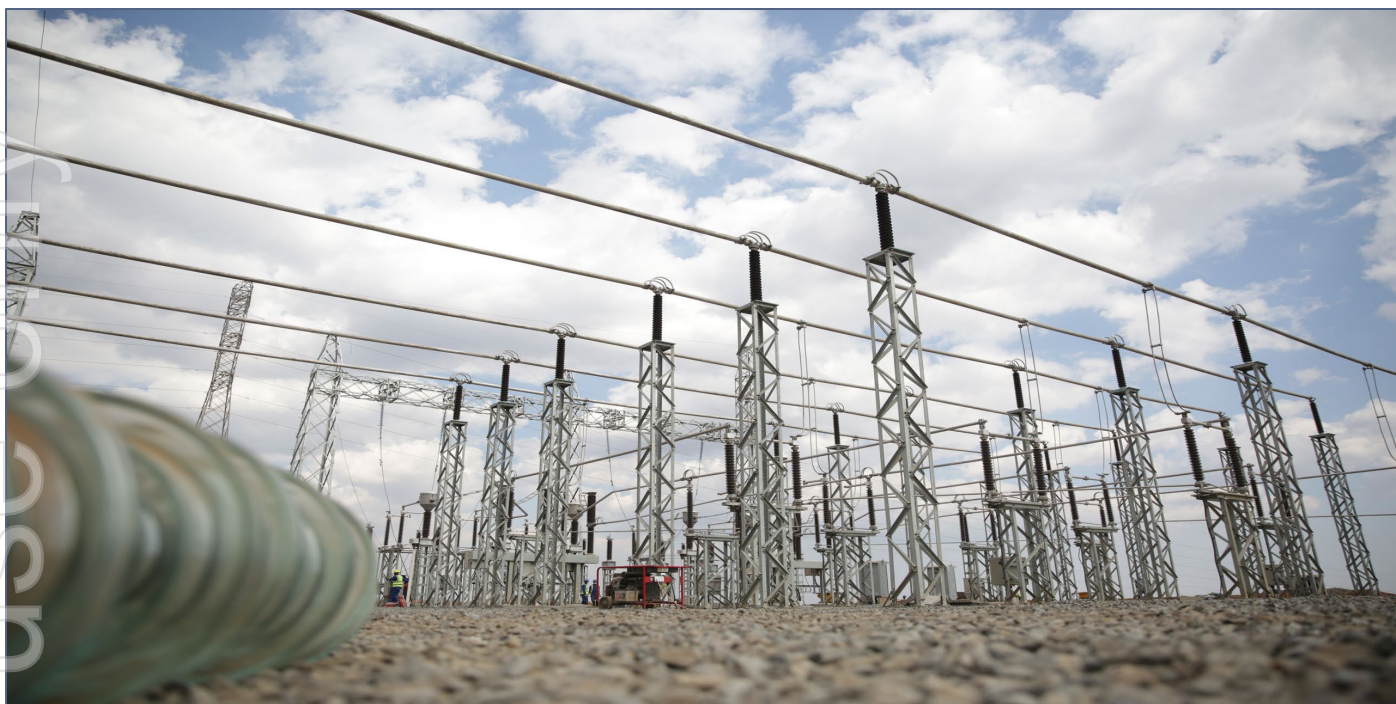
Figure 19: Nkhoma substation has capacity for connection to the Kasiya operation (Source: Millenium Challenge Corporation, USA)
