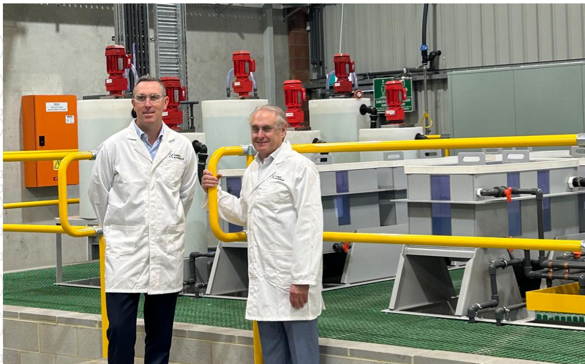
Figure 2 – Pictured ChemX CEO Peter Lee with Honourable Senator Don Farrell, Special Minister of State; Minister for Trade and Tourism, Deputy Leader of the Government in the Senate inspecting ChemX's HiPurA ® Solvent Extraction (SX) module, still pending energisation infrastructure installation
