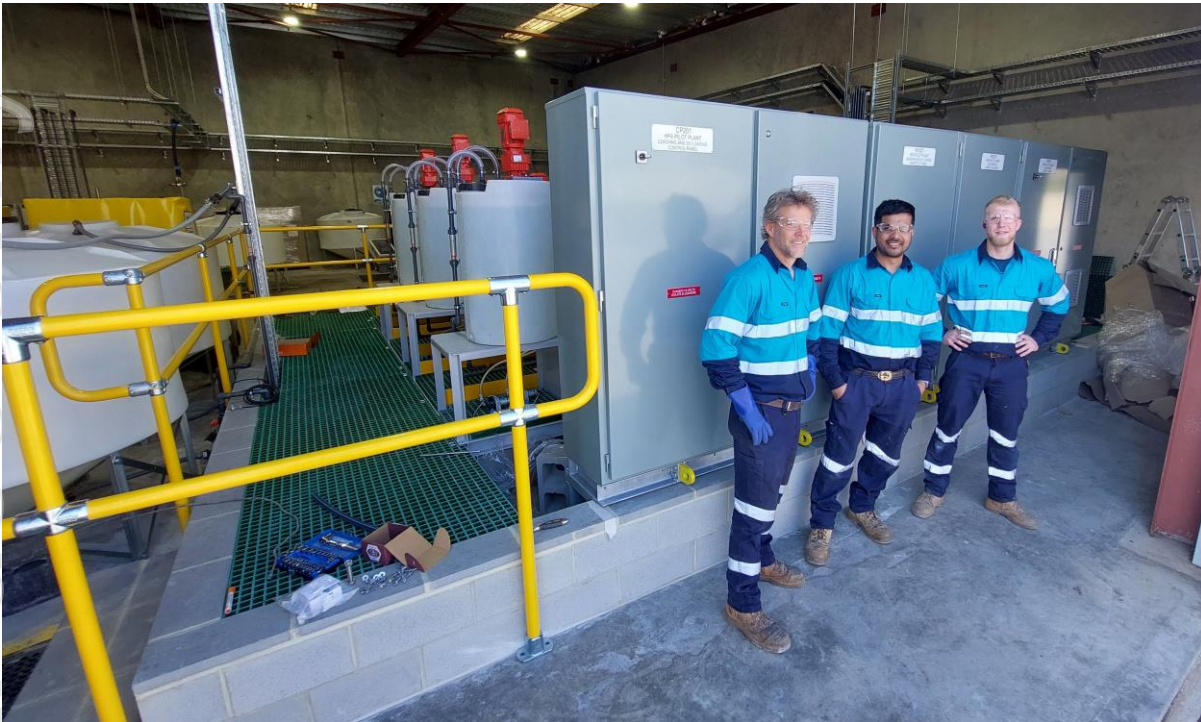
Figure 1 – ChemX Team pictured alongside the HiPurA® SX electrical control cabinets following successful installation
