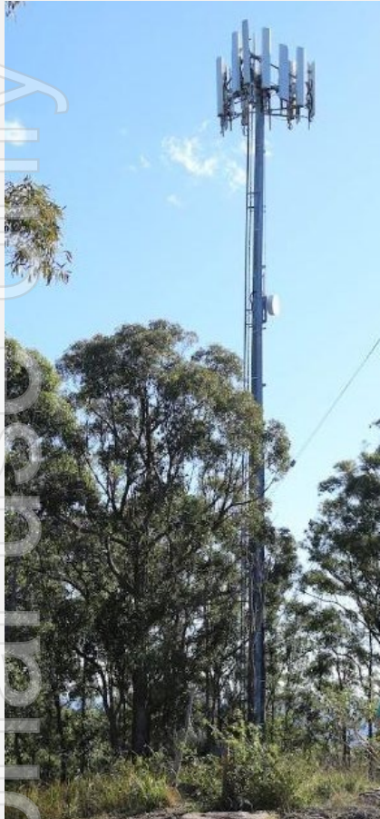
Securing mobile tower access
