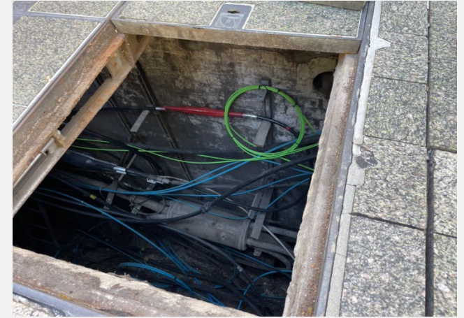
Protection of communication pits
