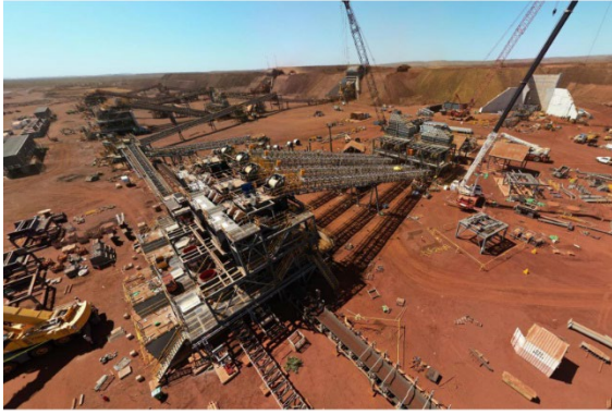
Three crushing trains at Ken's Bore
