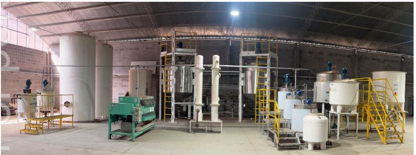
Figure 6: 250tpa Lithium Carbonate Plant at Pursuit's purpose facility in Salta, Argentina
