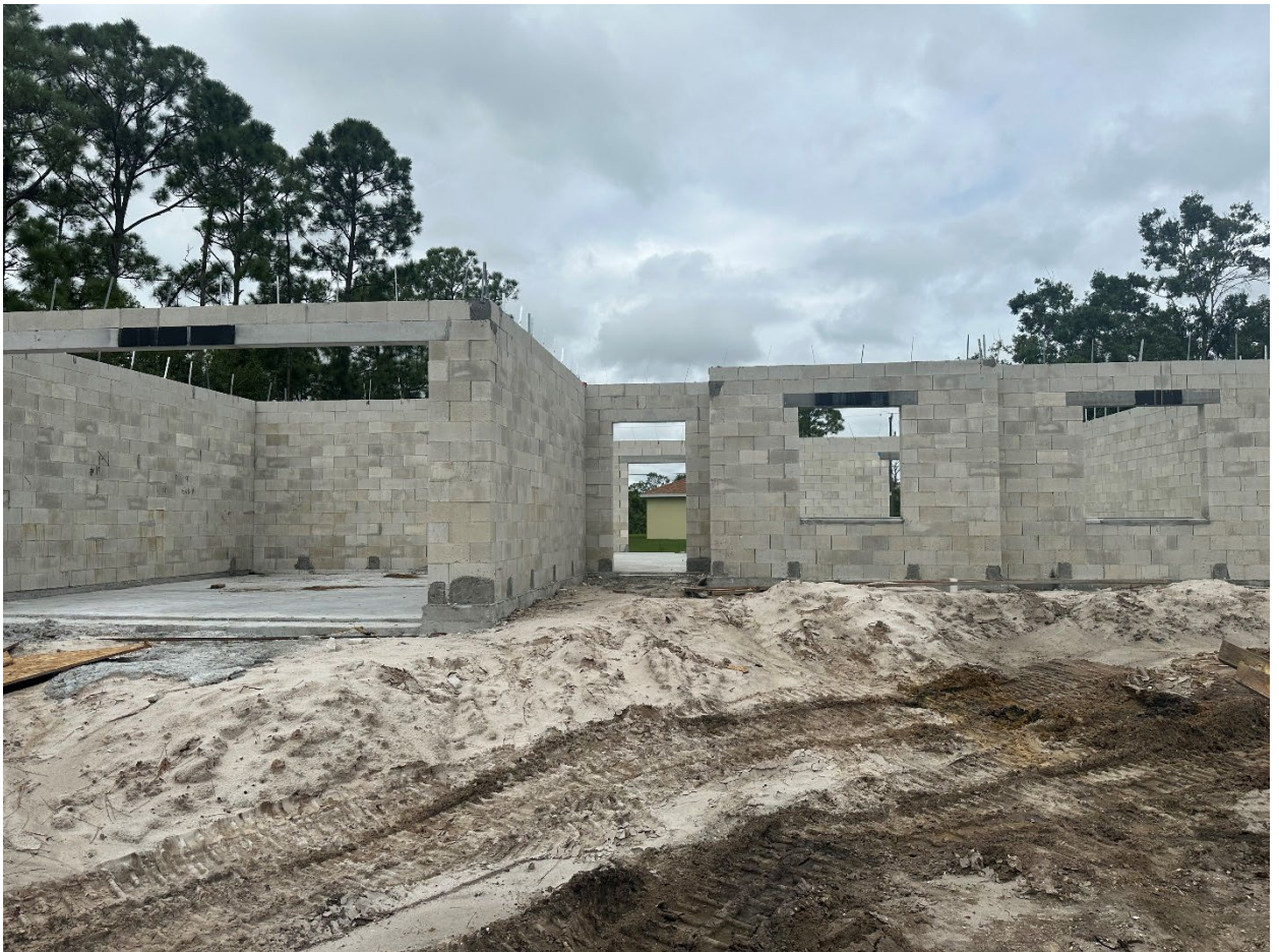
Pictured: A post-storm check of one of the houses built in the Demonstration Program in Florida
