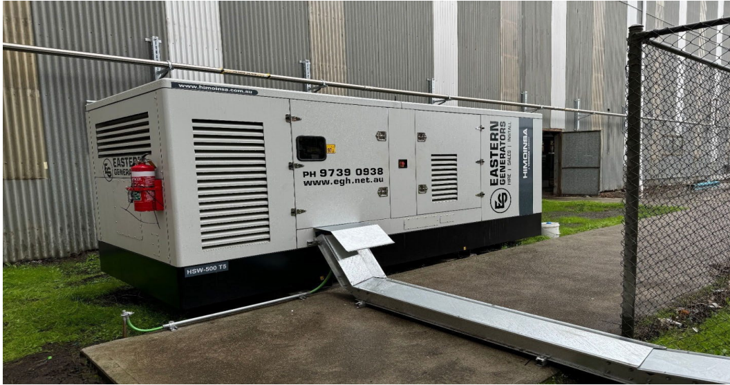
Emergency Standby Generator installed
