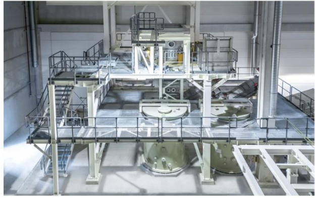
Figure 5 – Part of the Integrated LiB Plant installed by Primobius.
