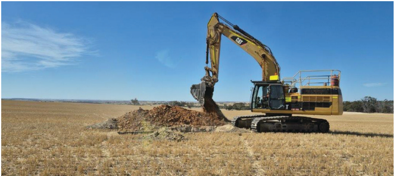
Figure 10 – Excavator digging a geotechnical test pit beneath the planned Tailings Storage Facility
