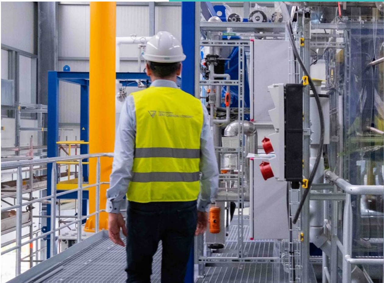
Process Mezzanine at Vulcan's CLEOP.
