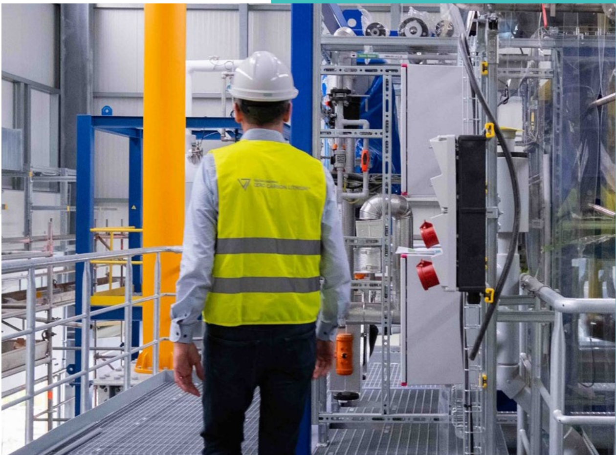
Process Mezzanine at Vulcan's CLEOP.
