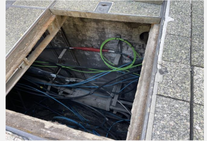
Protection of communication pits
