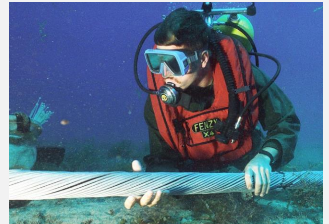
Monitoring of subsea telco cables
