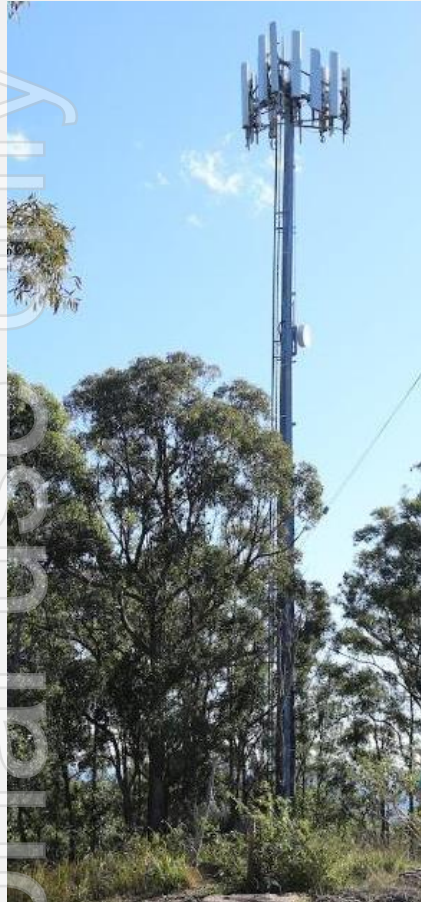
Securing mobile tower access
