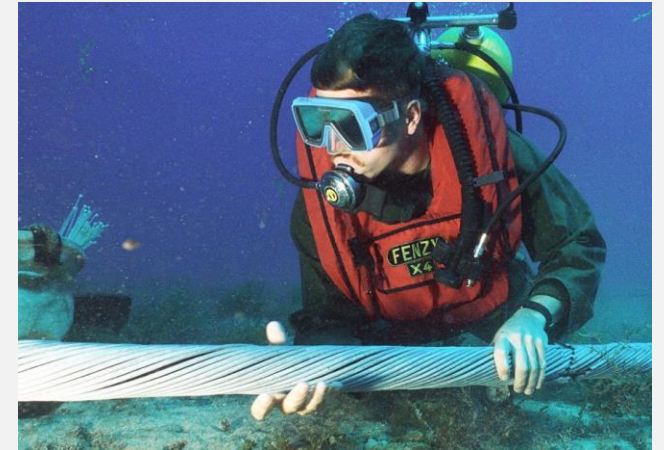
Monitoring of subsea telco cables
