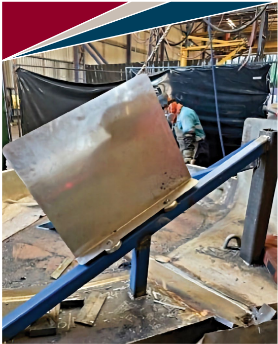
Aluminium welding screens
