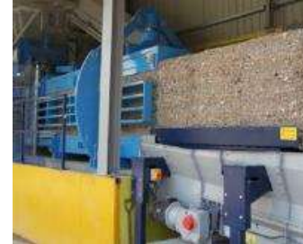
Waste to Energy
