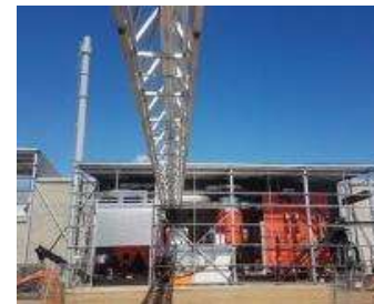
Biomass Steam & Hot Water Generation
