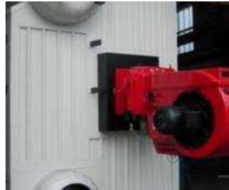
Industrial Steam Boiler
