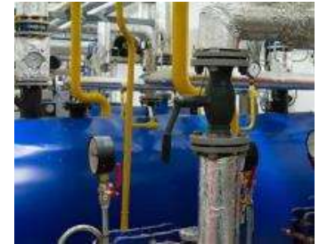
Large Commercial Hot Water Boilers
