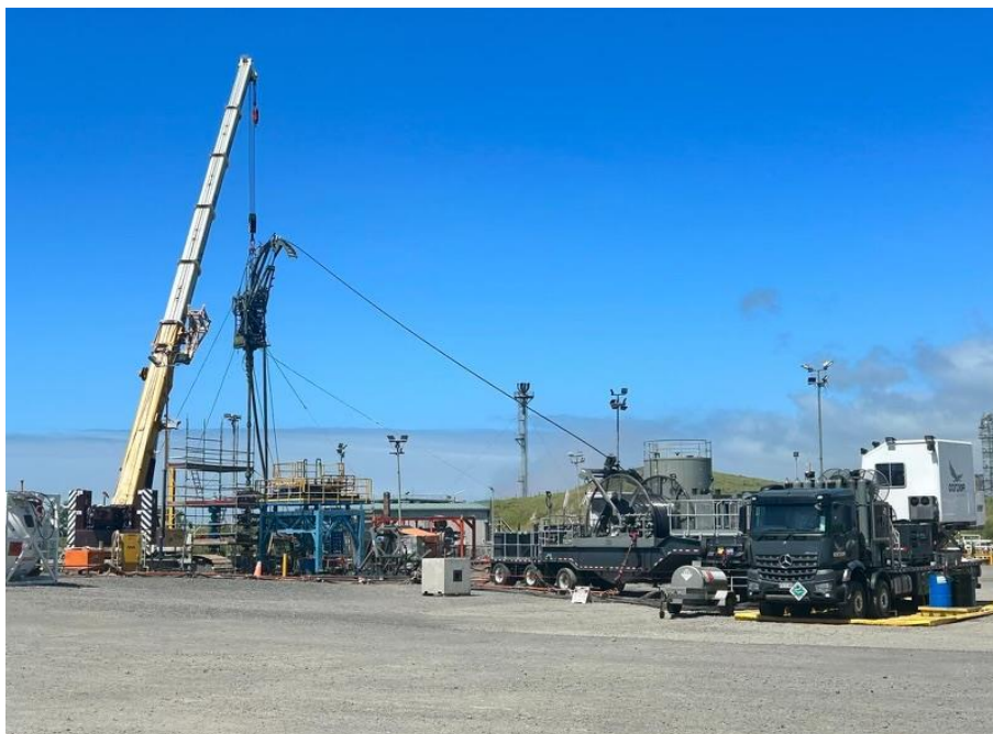
The CTU operated by Condor Energy (on a previous well location)
