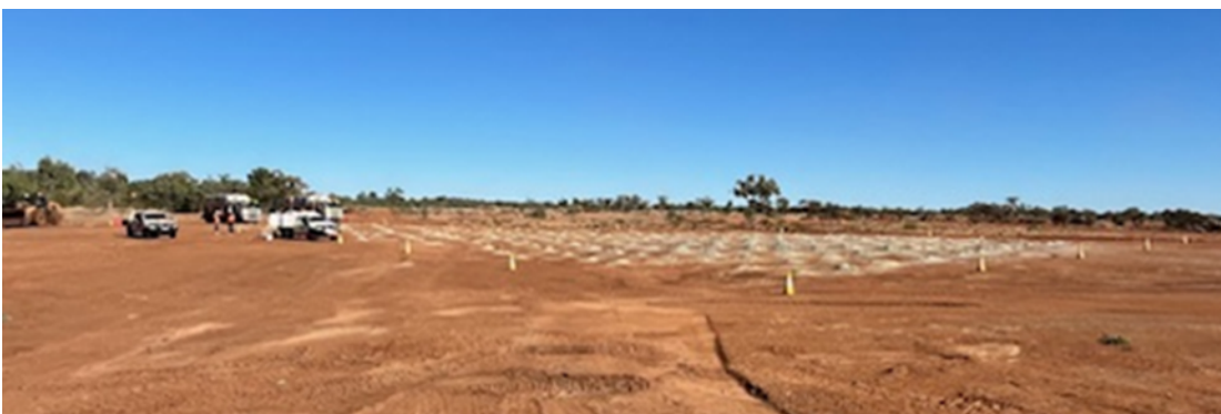
Figure 1 & 2: The 1st Blast shot being loaded in readiness for firing at Wallace North
