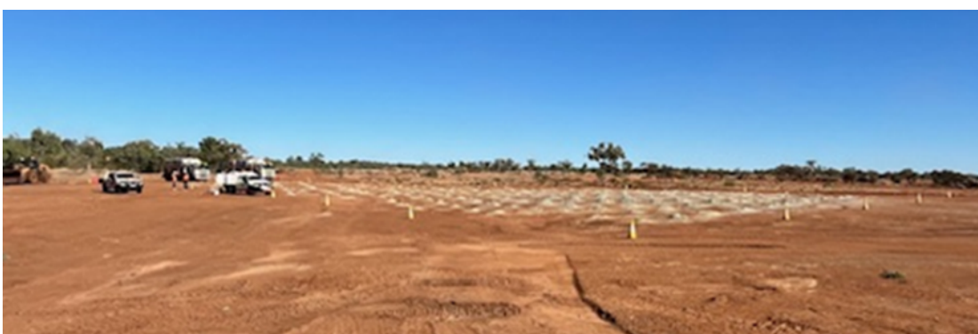
Figure 1 & 2: The 1st Blast shot being loaded in readiness for firing at Wallace North
