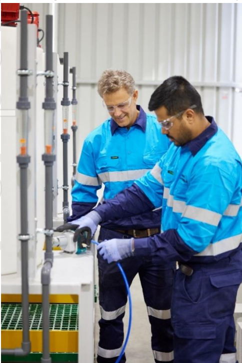
Figure 2 - ChemX Team actively plumbing key reagent delivery systems to the unique HiPurA® SX Circuit
