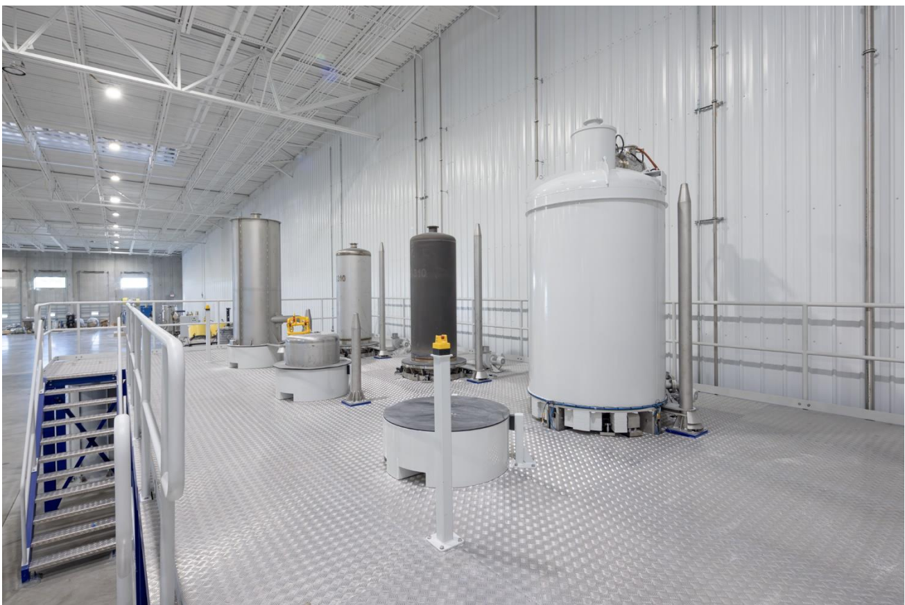
Figure 1: IperionX’s HAMR furnace deck, with site acceptance testing underway at the Titanium Production Facility
