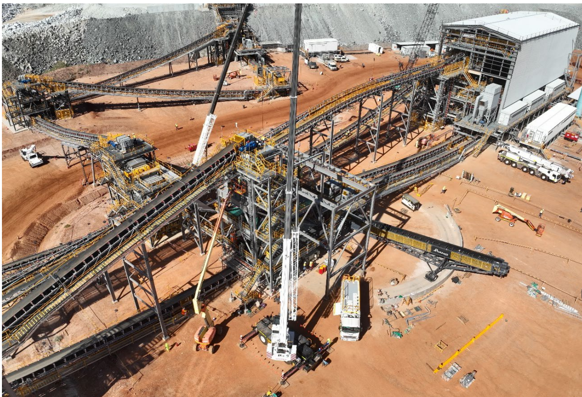
Figure 1: The P680 crushing and ore sorting facility as at 15 July 2024.
