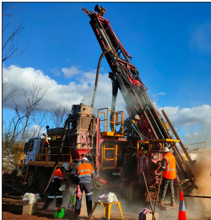
Photograph 1 –RC drill rig set up on the first planned drill-hole to test the 1.2km trend of spodumene-bearing pegmatites to the southwest of the Medcalf Spodumene Prospect (see Figure 2).
