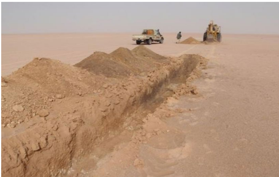
Figure 5: Typical landscape within Tiris project area, trench illustrating soft sandy overburden with gravelly free digging calcrete ore generally less than 6 metres deep.
