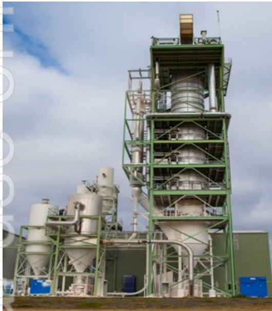
Bacchus Marsh Commissioned 2013 (50,000 tonnes per annum 1 )
