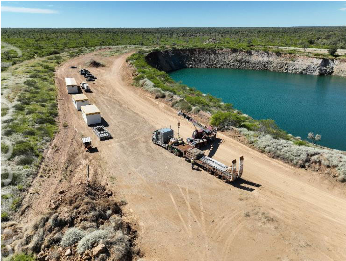
Figure 5. Wallace North office, workshop and fuel facility preparation adjacent to water source at Wallace South Pit. Image taken 23 April 2024.
