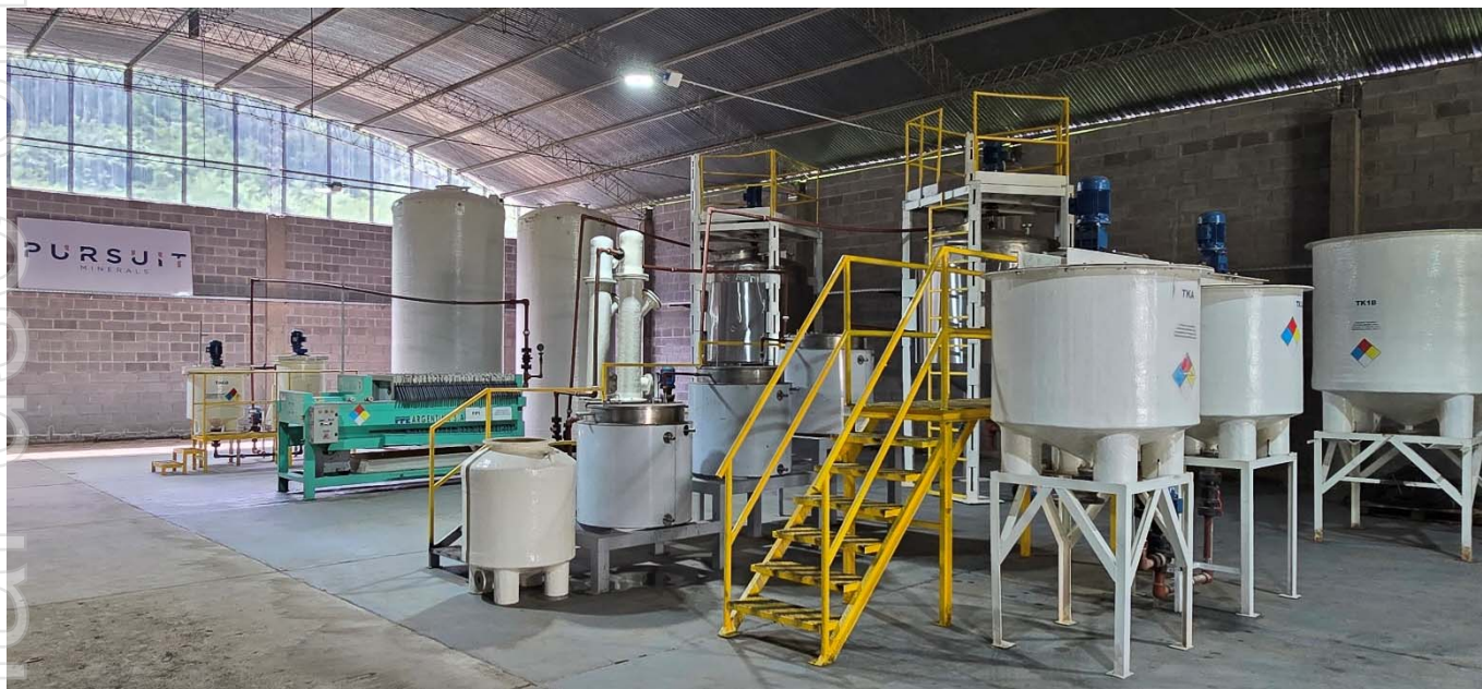
Figure 7: 250tpa Lithium Carbonate Plant at Pursuit's purpose facility in Salta, Argentina
