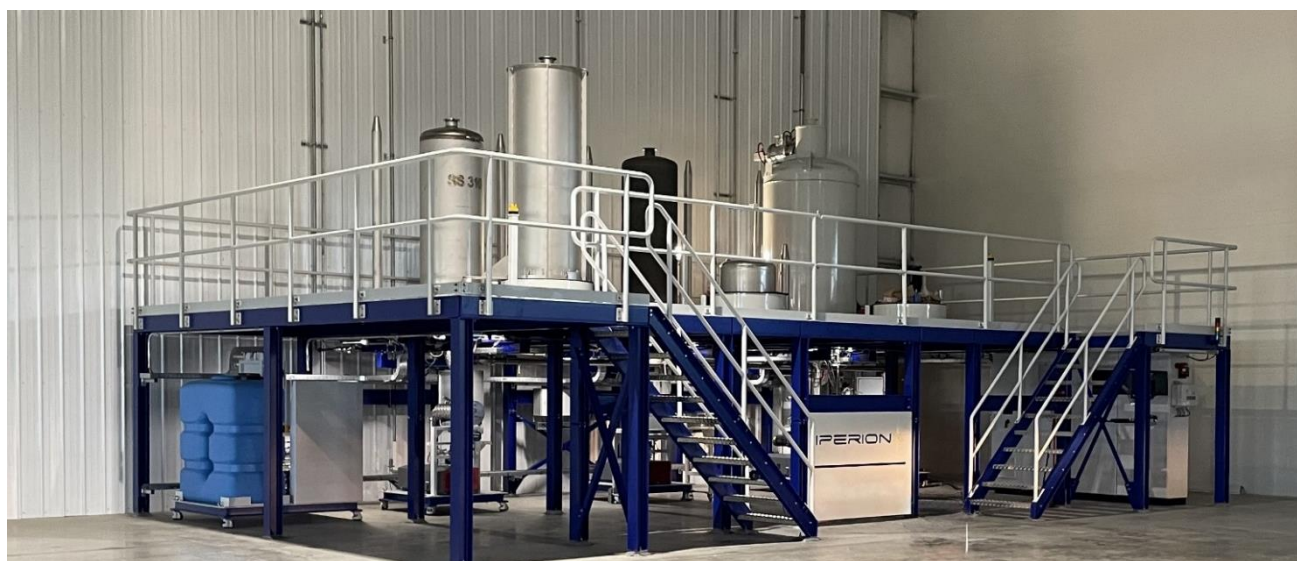
Figure 1: HAMR titanium furnace installed at the IperionX Titanium Production Facility
