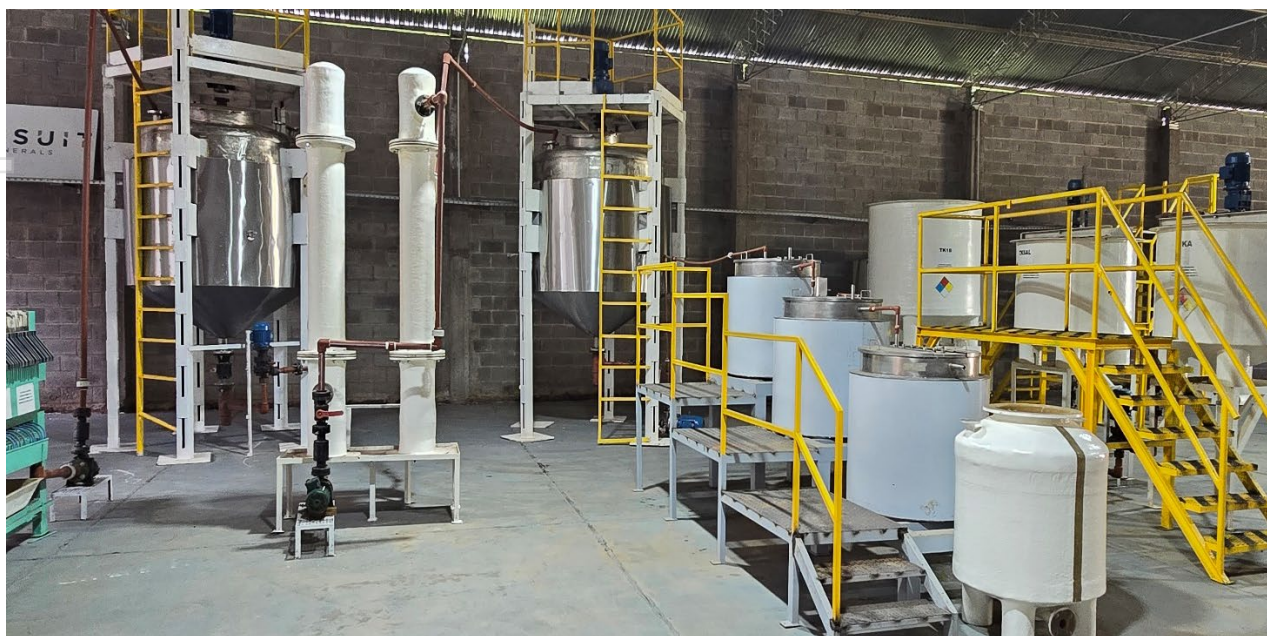
Figure 1 – 250tpa Lithium Carbonate Plant at Pursuit’s purpose facility in Salta, Argentina.
