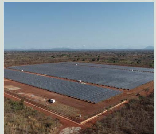
Balama solar and photovoltaic array
