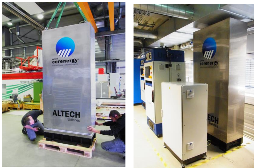
Figure 31 - Delivery of the battery casing and heat loss testing at Fraunhofer IKTS Dresden
