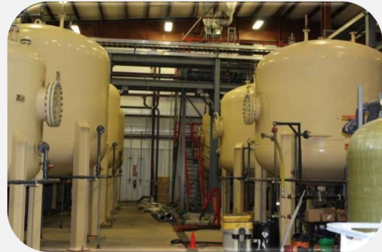
Lance Satellite Plant Ion Exchange System
