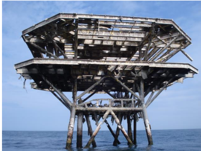
Figure 2 – C-18X well platform
