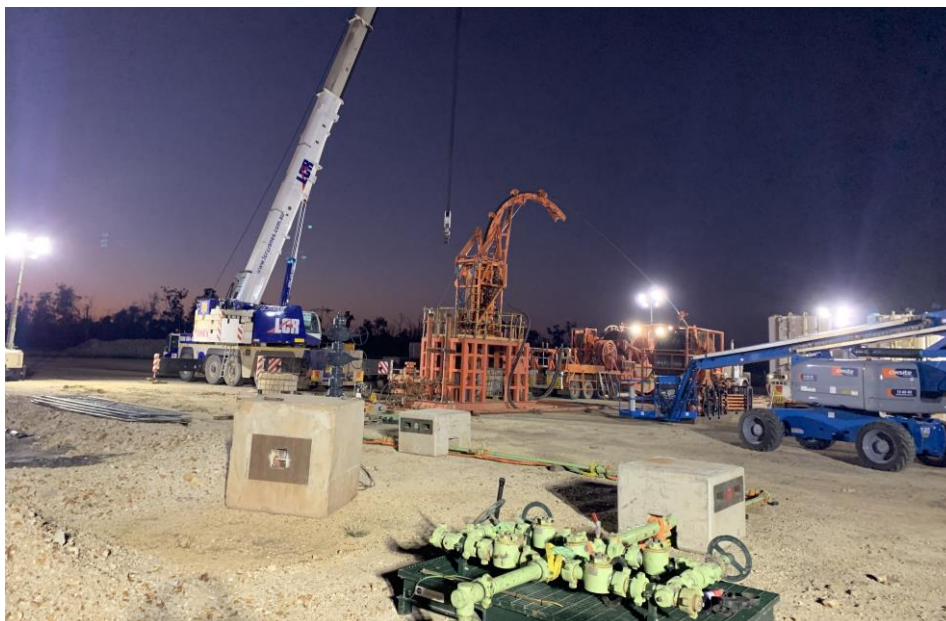
Coiled tubing unit at Daydream-2
