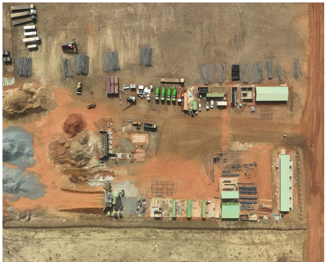
Figure 14 – Concrete batch plant at Kiaka
