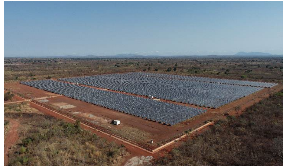
11.25 MWp solar photovoltaic array
