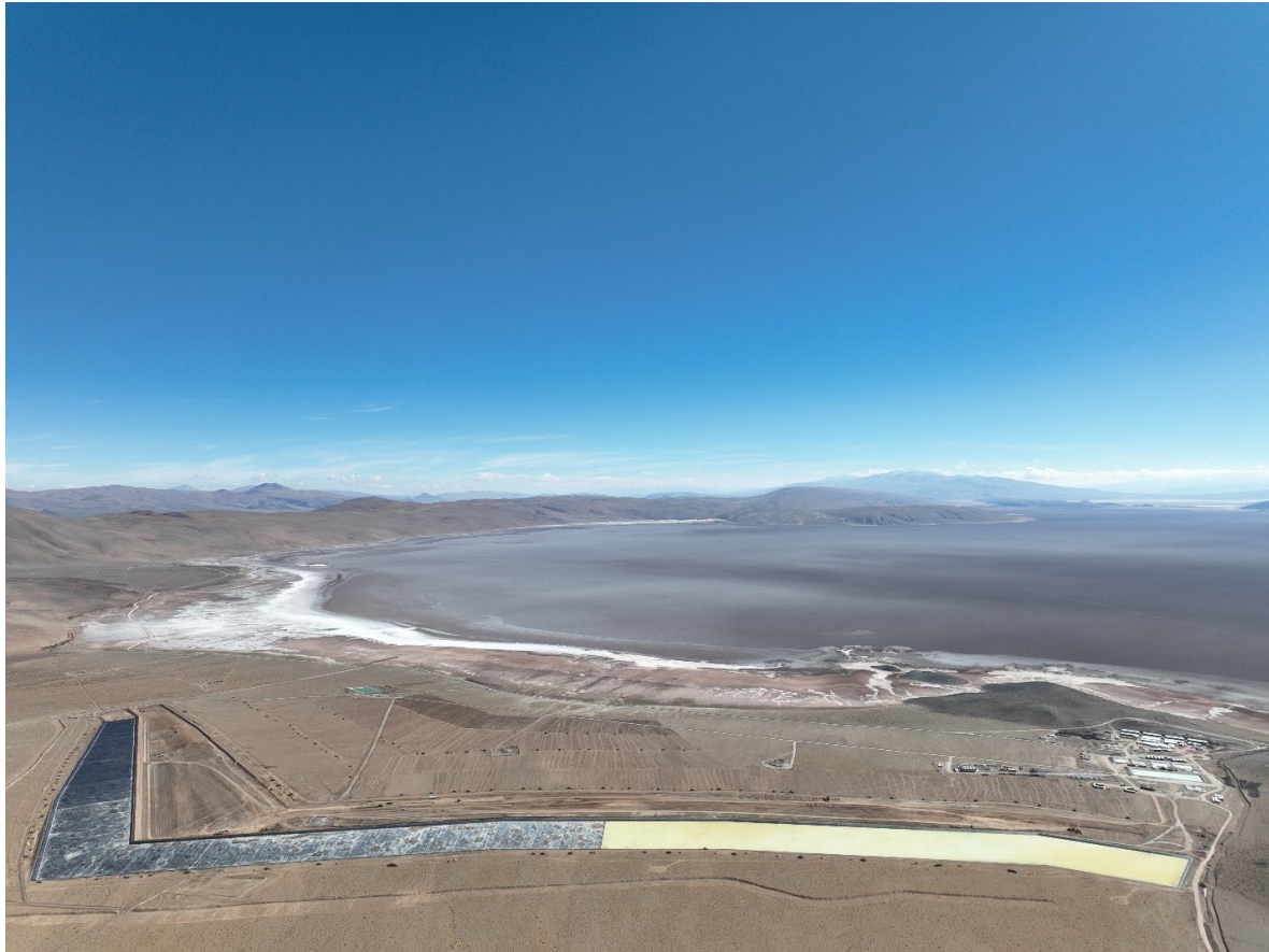
Completed liner installation on Pond (evaporation commenced) and progress of Pond 2 construction 2
