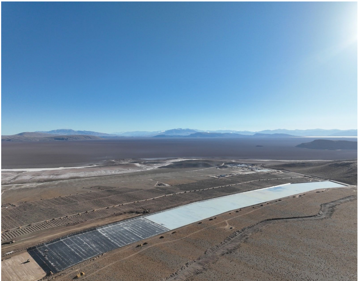
Figure 2 – Overview of HMW Phase 1 project construction with the filling of Pond 1 in the foreground
