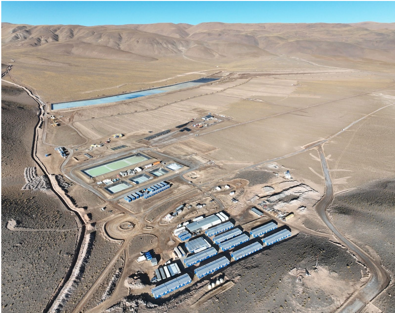
Figure 1 – Overview of HMW Phase 1 project construction (includes camp, pilot plant and filling of Pond 1 in the background)
